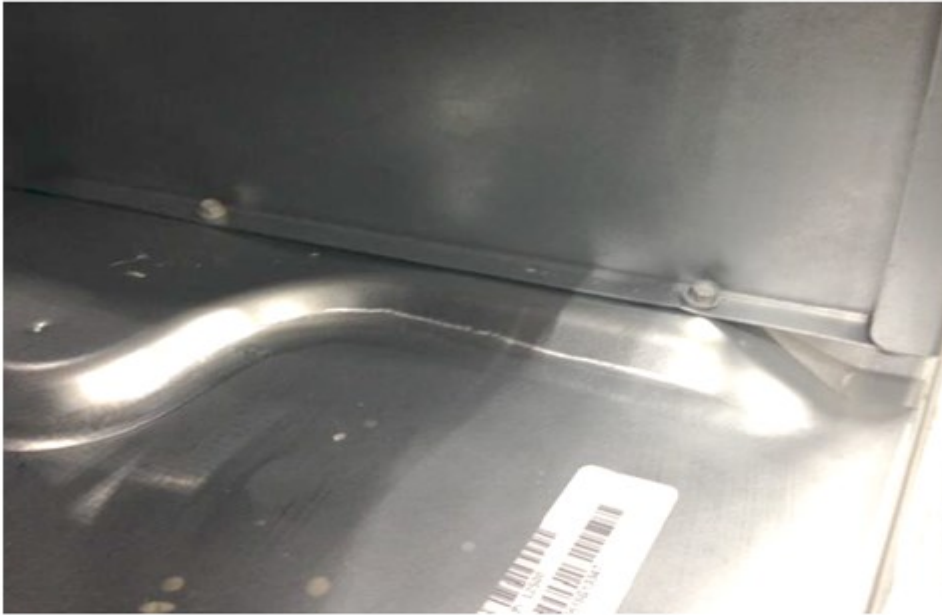
Condenser side of the removable panel.
